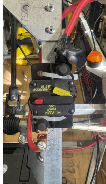
(b) 120 A main breaker.
